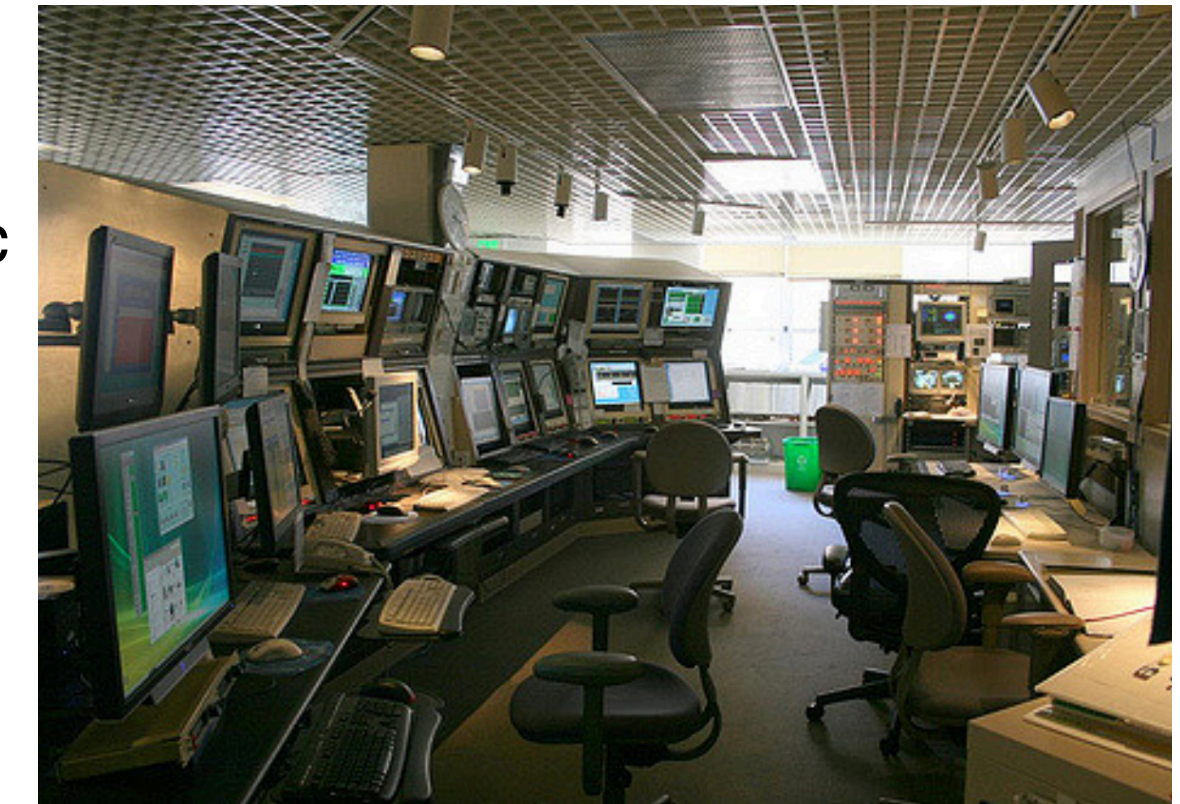
High level controls
